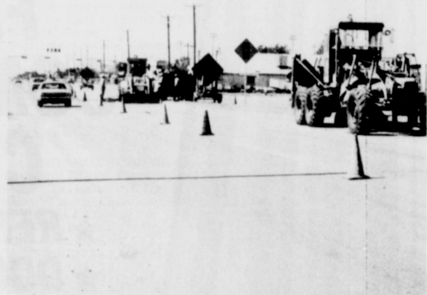
ROAD WORK...A crew from the highway department was in Friona this week making repairs to the roadway to the east of the Main Street intersection.
