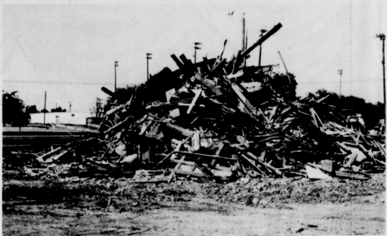
FORMER RESTAURANT...Demolition work was completed this week at the former location of the Holiday
