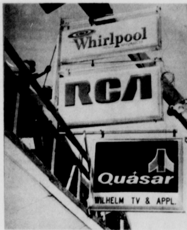
NEW SIGN... Workmen are shown installing a new sign at Wilhelm TV and Appliance. The Wilhelms have also added some display fixtures inside their Main Street store.
