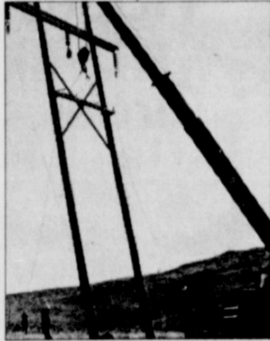
"We're putting in a new 115,000 volt line . . . gives us another feed to back up our dependability . . ."
