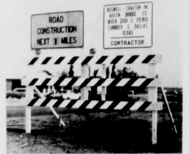
ROAD SIGNS...Signs proclaiming the pending construction on State Highway 214 have been erected at the start of the overpass section, on South Grand in Friona. Actual dirt work for the huge bridge is expected to begin on Monday.
