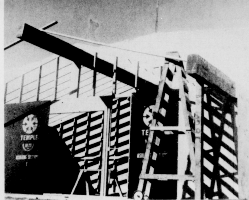
CONSTRUCTION ACTIVITY.... With perfect weather most of the past week, outdoor activity really picked up. Three different construction sites are shown in these photos. At the top is a residence in the Western Addition. Center photo shows the addition to Friona Country Club. At bottom is the foyer which is being added to the new Community Center-Show-barn. [Star Photo]
