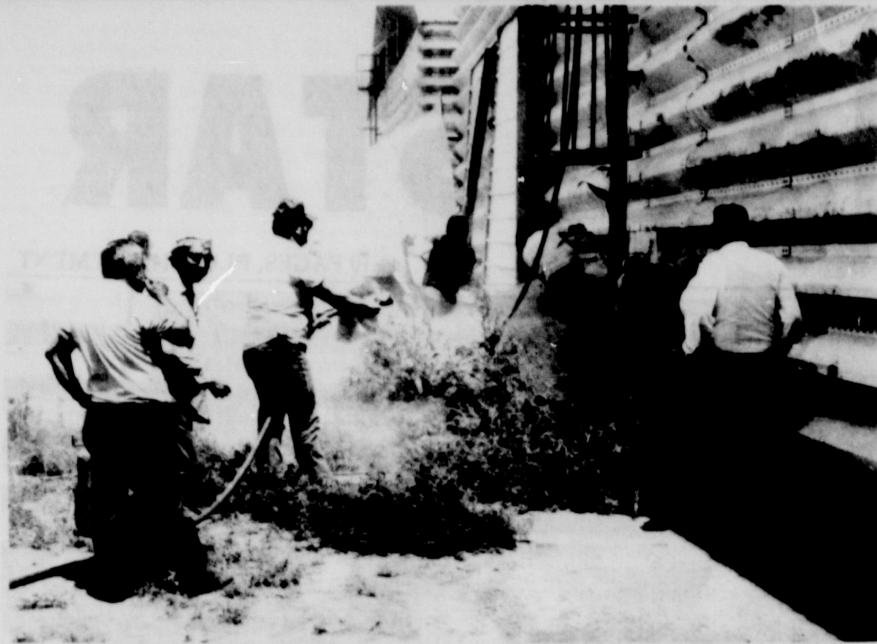
OPENING MADE.... Rescue workers are shown as they cut an opening in the steel grain bin at West Friona Grain Thursday afternoon. At the left center, Friona Fireman Beamon McDonald waits with water hose in case the sparks from the torch should set off a fire.
