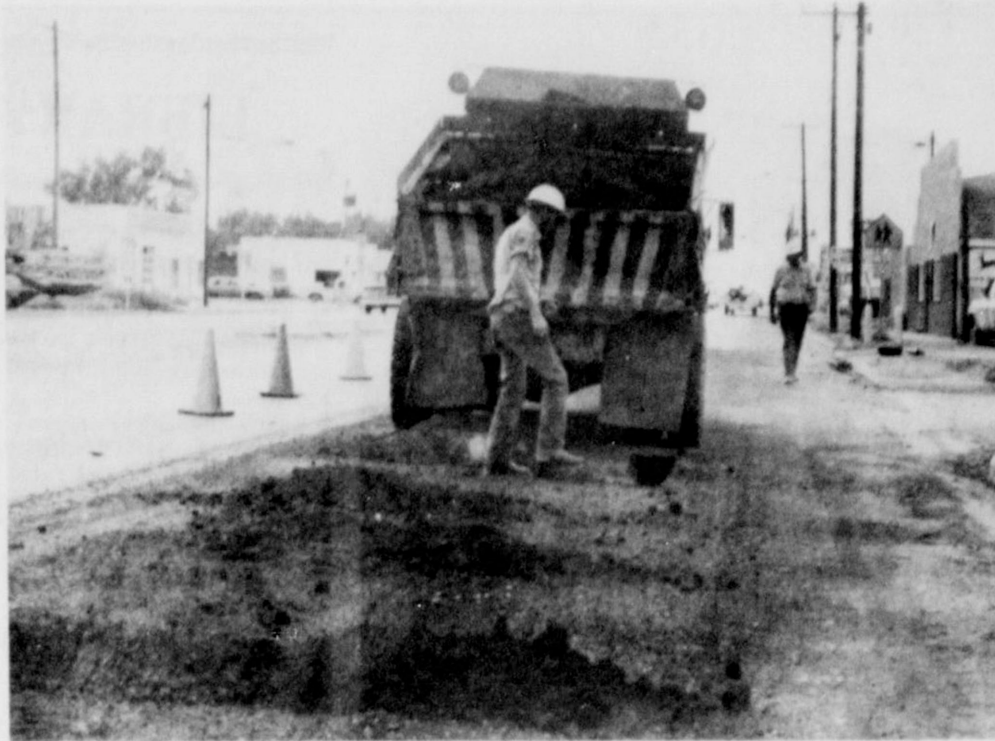
ROAD REPAIRED... Employees of the Texas Highway Department have been busy in Friona for the past few weeks making major repairs to Highway 60 through the city. Many sections of the highway have been
