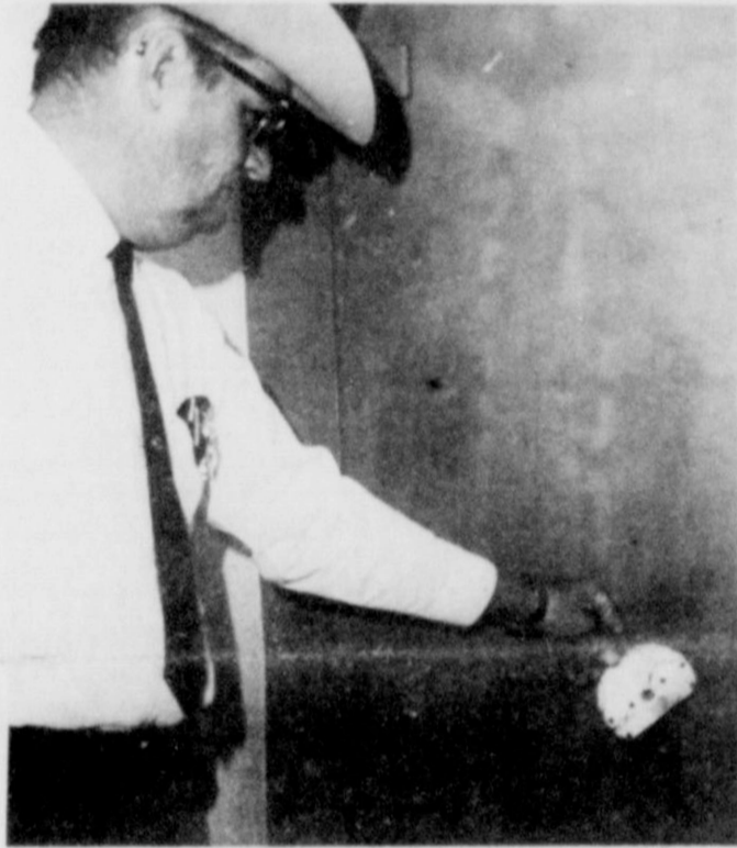
TAMPHERED SAFE AT HIGH SCHOOL...Friona Police Chief Bill Denney shows part of the dial which was knocked from the door of a vault at Friona High School Monday night. Although vandals knocked off the dials and tampered with the hinges, the vault remained unopened.
