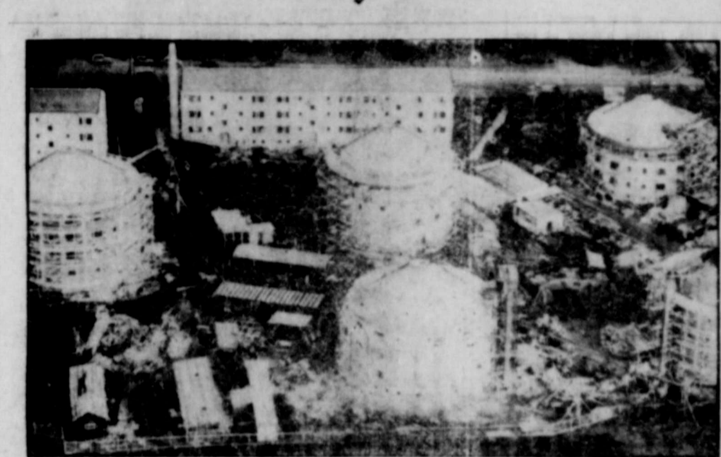
'ROUND THE FAMILY CIRCLE—These unique circular apartment houses are under construction in a Stockholm, Sweden, suburb. The new-type building contains 10 one-room apartments on each of their four floors, the rooms being placed fan-shaped around a large, circular staircase. Each of the houses will be painted a different color.
