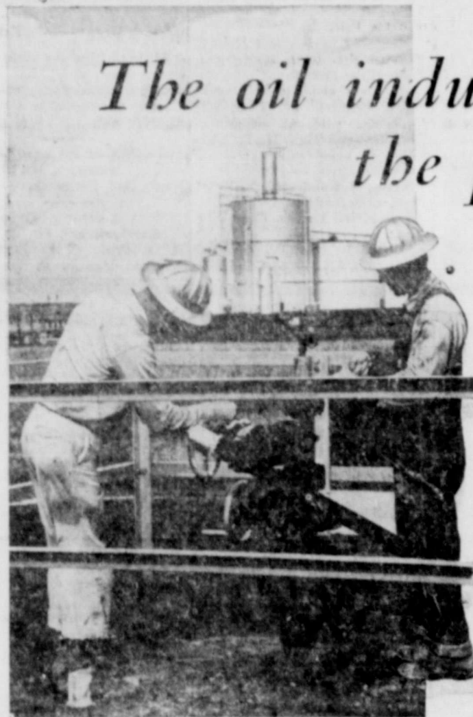
1. This is the "Christmas tree" you've heard oil men talk about. It is a complicated arrangement of valves and meters which regulate the flow of oil from a producing well. This well is on Humble's lease in the Conroe field in Texas.
