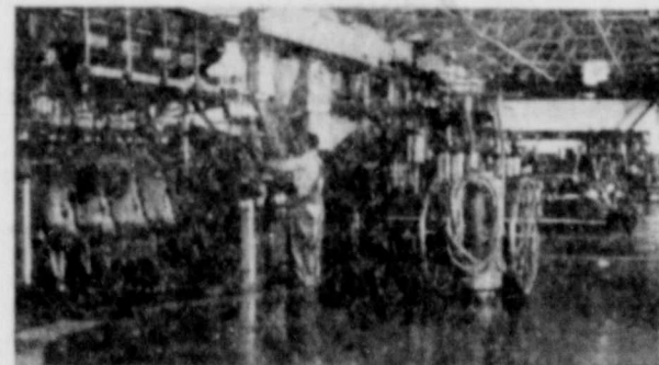
2. Oil pipe lines have worked wonders in oil transportation to carry your record demand for oil. This is the interior of Humble Pipe Line Company's pumping station at Comyn. This company operates 8,703 miles of oil and finished products pipe lines in Texas and New Mexico. Though construction of additional pipe lines has been slow because of the high demand for steel for other purposes, the Humble Pipe Line Company has been able to handle the largest volume in its history; during 1947, main trunk lines delivered 253,000,000 barrels of oil.
