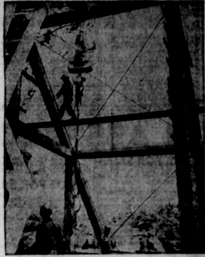
ARMY BUILDERS AT WORK—Where go the Army Engineers, a bridge is sure to follow. Here construction engineers of the Hawaii Army Reserve and the 65th Engineer Battalion build a 60-ton bridge—and a pattern for the Army photographer—on the East Range at Schofield Barracks, Hawaiian Islands.
