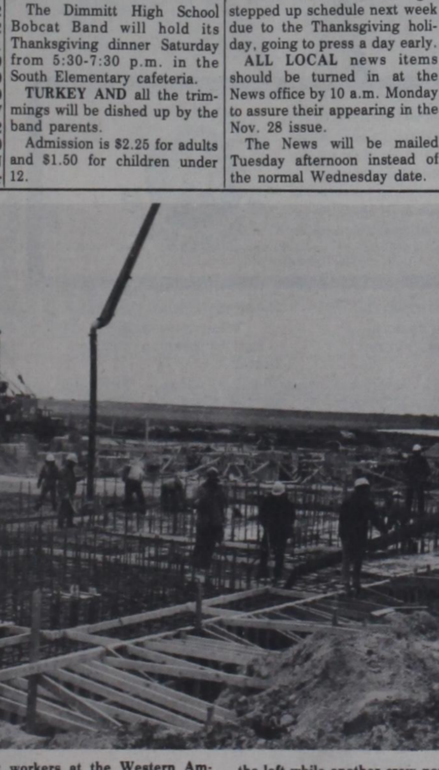
left while another crew pours the outer-wall area from the right. In background work progresses on the main part of the new plant, which is being erected south of the present plant site.
