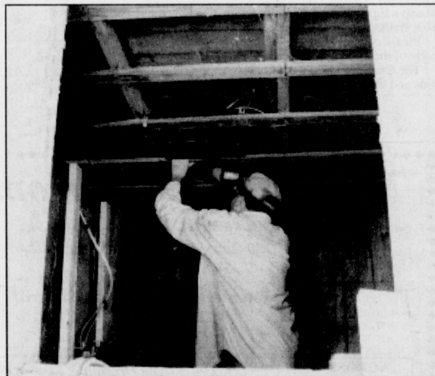
JASON YOUNG (left) and CRAIG GEHRELS work together to replace some wiring before the new ceiling is installed.
