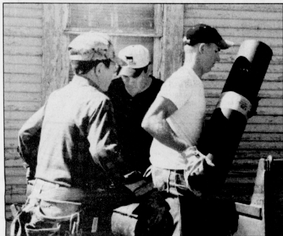
RAYMOND LINDSEY, JOE ESCALONA, & GUY SLIMP load roofing paper into the front loader bucket before they climbed on the roof.
