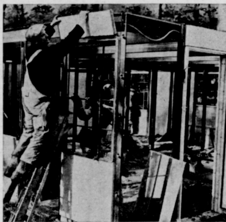
Workers put into place one of the panels over the window to complete a section of a wall in a "pre-fabricated" house. Ten of these "streamlined" modern homes are being built on government land at Greenbelt, Md., by private capital in co-operation with the government as a possible solution to the nation's housing problem. They are designed for a family with an income of $3,000 a year and with one or two children.
