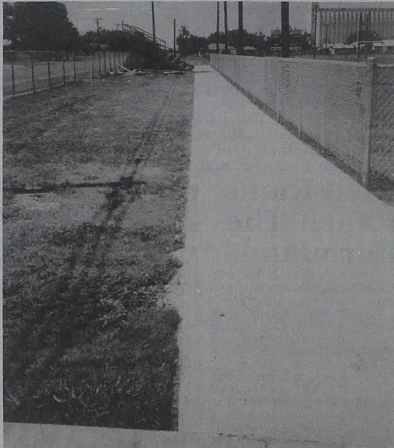
NEW VISITOR WALK..... Work was completed on a new sidewalk on the visiting team side at Mustang Field. The visitors bleachers were moved back to make room for the new walk and plans to refinish the visiting bleachers are under consideration.
