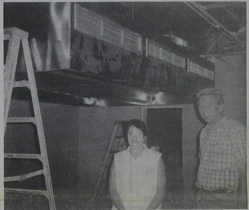
NO GREASE..... Cafeteria manager Cathy Riley and construction manager Mike Green newly installed vent-a-hood in the kitchen area of the cafeteria. With school starting in less than two weeks, workmen are hurrying to have the cafeteria ready for the students.
