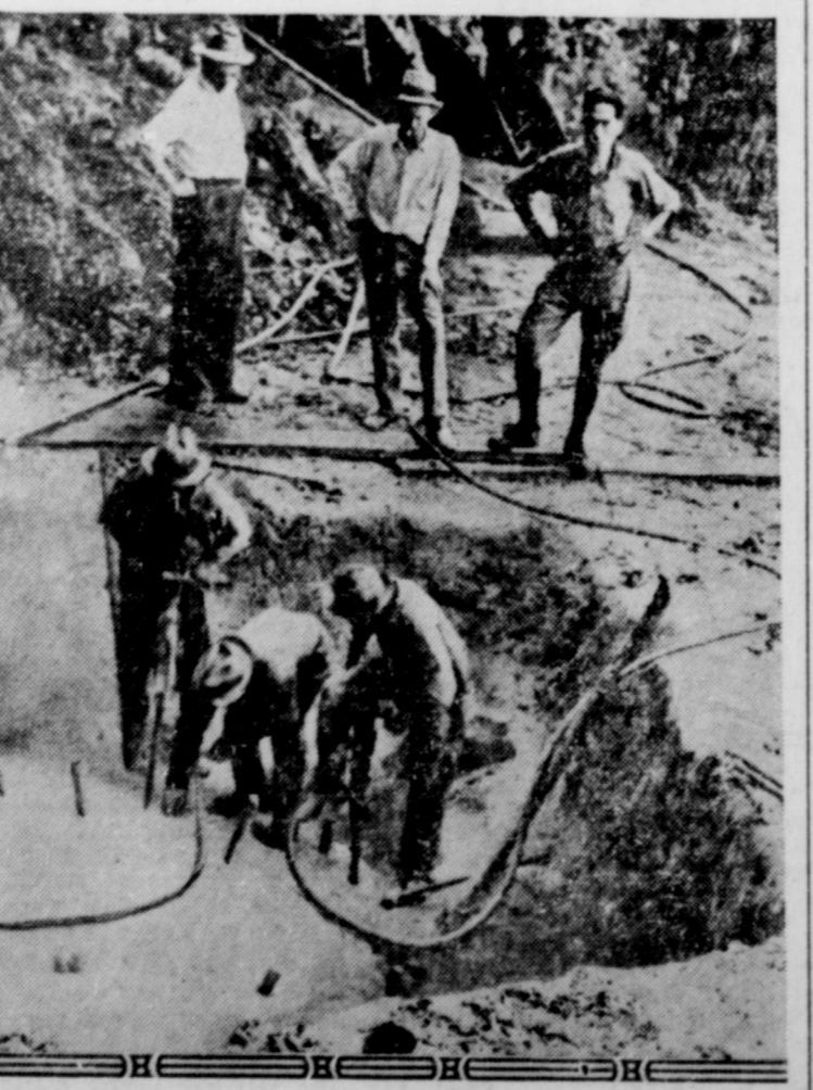
Workers at Cove Creek, Tennessee, preparing a shaft site for the first charge of dynamite as construction was commenced on the new Norris dam. The 100-foot shaft when completed will be used as a gauge of the dam foundation. The project, located on the Clinch river 80 miles above the point where that tributary joins the Tennessee river, will be joined to the Wilson dam at Muscle Shoals by a 220-mile long tie-transmission line.
