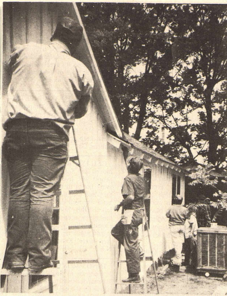
WORKING HARD - Sooner or "ladder" the Christmas in April project will be all done after workers finish this paint job.
