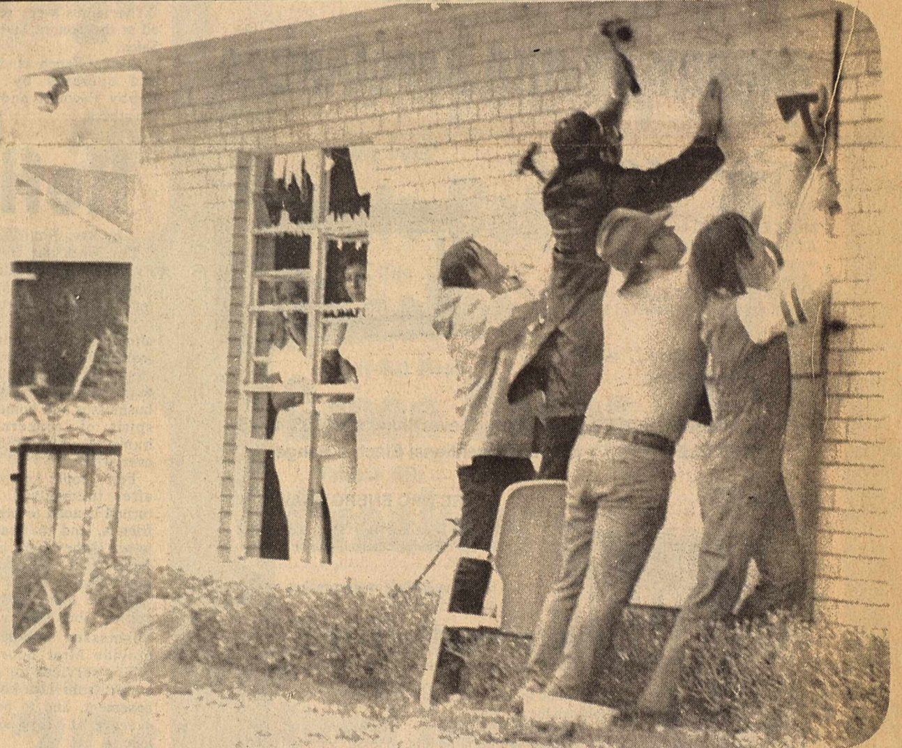
Immediately following the let-up of nature's hostilities last Friday, repairs were started on damaged buildings. High on the priority list was Hudspeth Memorial Hospital and the adjoining nursing home. Shown stopping up holes on the northwest corner of the home are from left, Everette Adgborn, Rev. Jim Miles, Carl Weaver and Pat Campbell.
