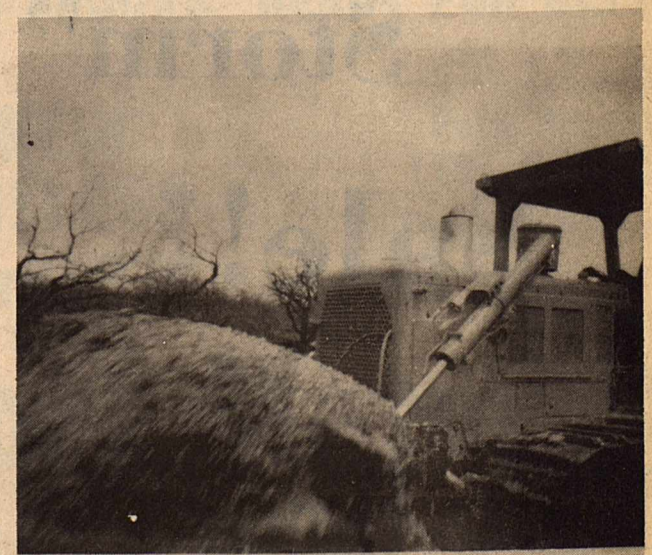
More dozer work--in some outlying areas, hailstones were piled up to depth of two and one-half feet on the county roads, and the County was forced to hire both equipment and operators in order to clear the right-of-way.
