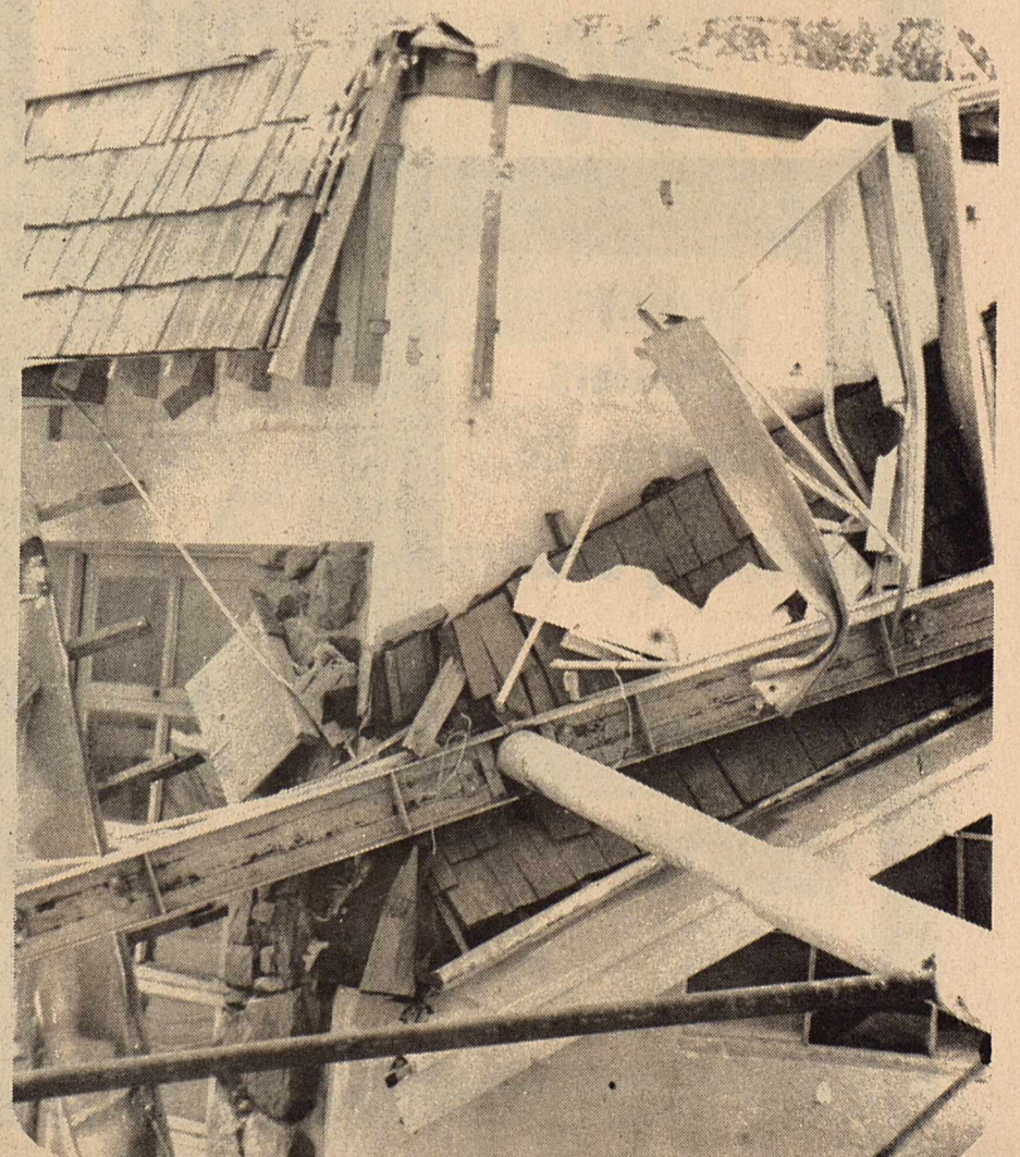
More wind destruction is shown at Jim Green's Texaco Service Station on Crockett. The debris above is the result of the tall sign close to the station being blown into the building itself, resulting in structural damage to the station proper. [Photo by Kay Holdridge]
