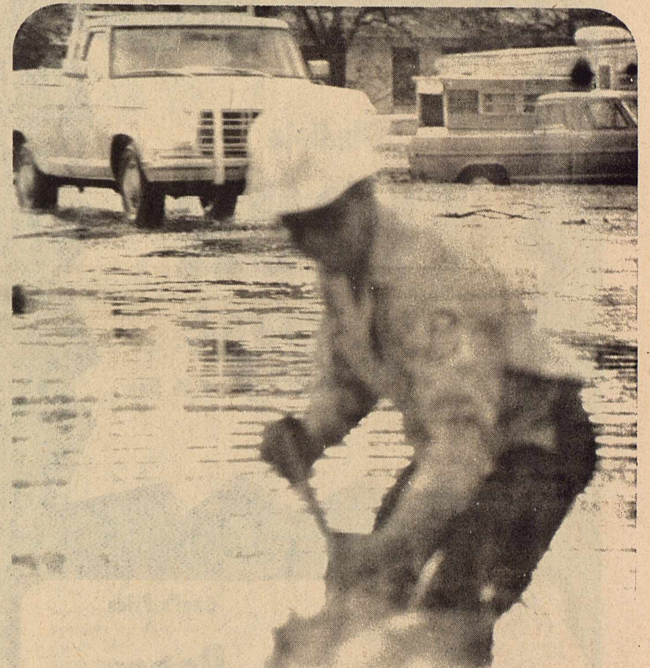
A City of Sonora employee making an effort to clear rocks and debris, or at least to divert the flow of water on Concho, just north of the former railroad tracks.
