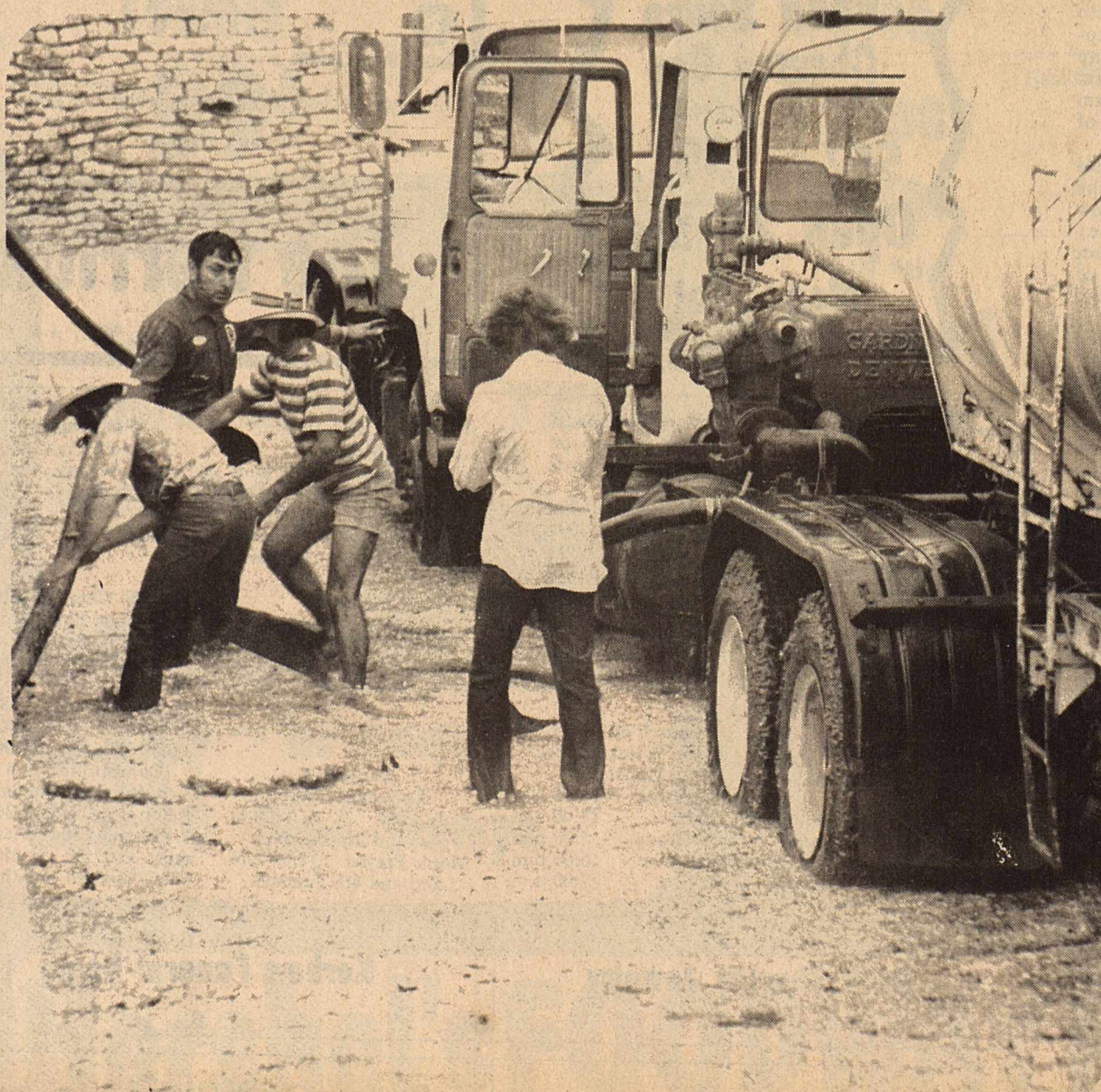
Hudspeth Memorial Hospital was hard-hit in the recent severe storm. Shown pumping water from the hospital's flooded basement are Pool Company employees Jimmy Fiveash [holding pipe], Pete Aguero, Sam Barbero and Kippy Joiner [with back to camera]. They are among many who helped during the emergency.
