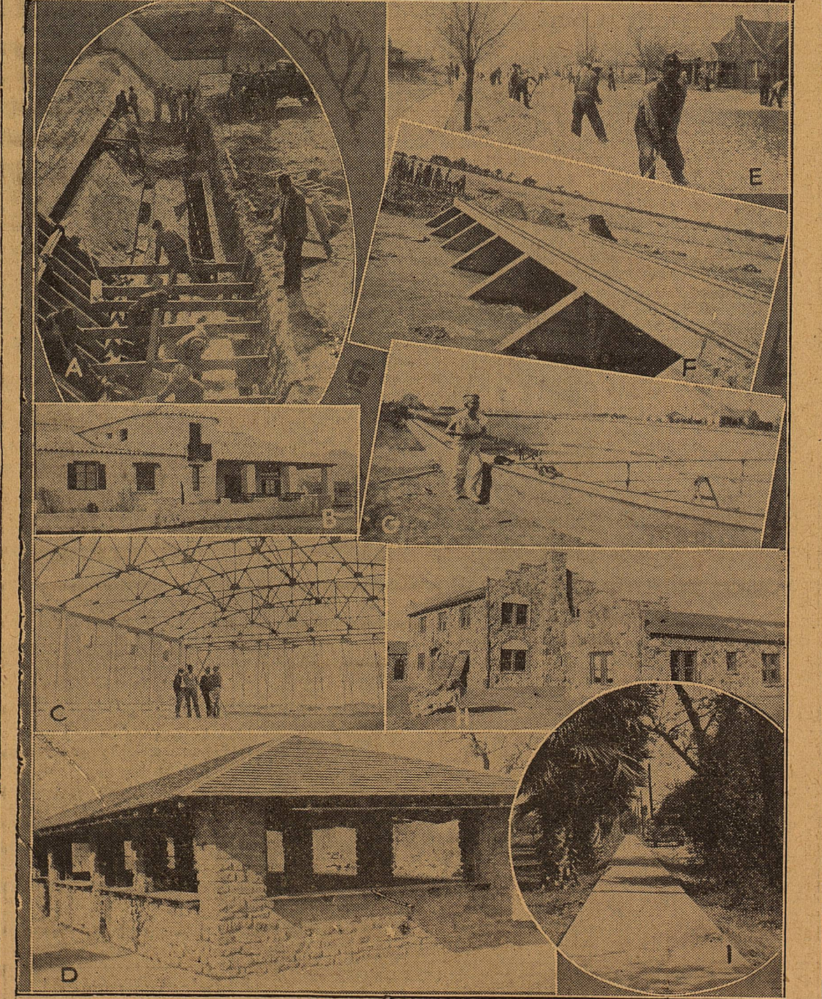
(A) Complete repairs of flood damage to the Lake Trammell dam, vital link in the water system of the city of Sweetwater, were effected by WPA laborers. (B) El Paso's beautiful new municipal golf building was recently completed by WPA workmen as part of the project which provided thorough improvement of the city course. (C) A hangar for one of the 12 airports being built by WPA in Texas is seen here in the process of construction at Fort Stockton. (D) This attractive, native-stone concession house is one of several permanent buildings included in the project which improved 194 acres to create a park at Lake Brownwood, four miles from the city of Brownwood. (E) Workmen spread rock on the first course of asphalt in the Lubbock street-paving program. (F) This concrete low-water bridge, constructed by WPA workmen, now spans the Nueces River ten miles southwest of Uvalde. (G) Chillicothe's new municipal swimming pool provides a recreational center highly popular with citizens of the town. The pool is 60 by 125 feet in size. (H) This handsome meeting house and its surrounding cottages comprise Buffalo Courts, attractive and comfortable dormitories for students at West Texas State Teachers College at Canyon. Low rentals charged by college authorities for these accommodations make attendance possible for many youths who otherwise might be denied educational advantages. (I) A stretch of newly-constructed sidewalk enhances the attractiveness of McAllen streets due to WPA efforts.
