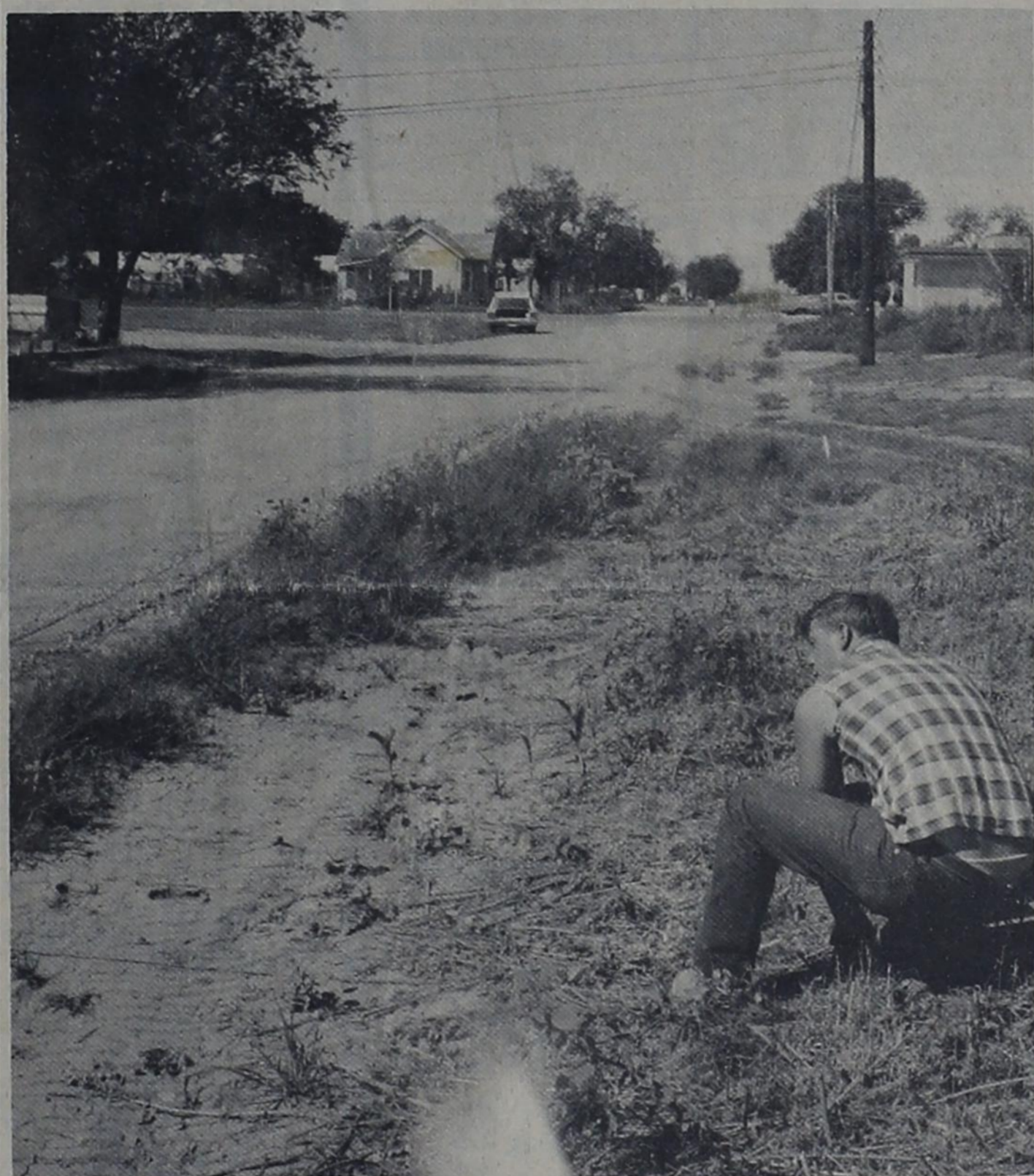
PAVING PREPARATION -- Bovina's forthcoming paving project is being staked out last week and this by an engineering crew from Lubbock. Determining the proper place for a stake on Avenue A is Darrell Jenkins of Lubbock. The staking work began the latter part of last week and is expected to be completed this week with the paving, curbs and gutters to be installed soon thereafter. The project is scheduled to include some 20 blocks.
