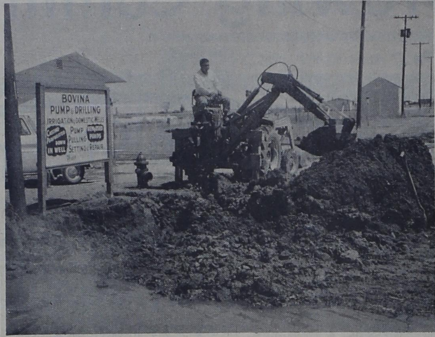
DIGGIN' FOR WATER -- City employee Andy Garza operates the city's backhoe in an effort to find a leak in one of the main water lines of Bovina. Water in the foreground flooded both sides of the Pleasant Hill highway before water was shut off here Tuesday morning.
