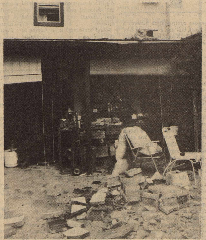
Lightning struck the chimney at the home of H.C. and Estha Barker, causing fire and scattered debris.
