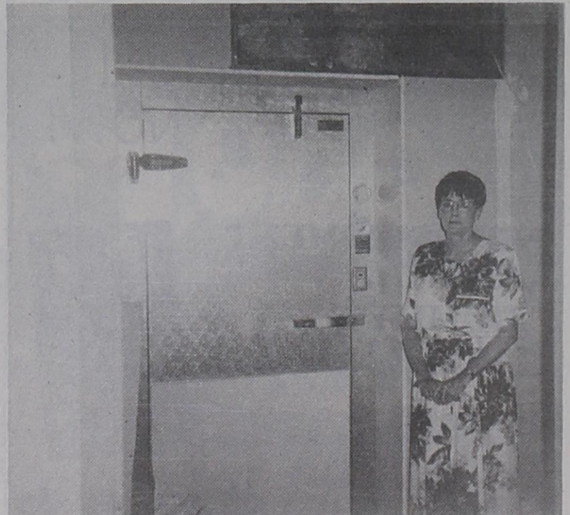
COOLER NOW..... Superintendent Sue Nuttall is showing off the school's new cooler and freezer installed during the cafeteria reconstruction this summer.
