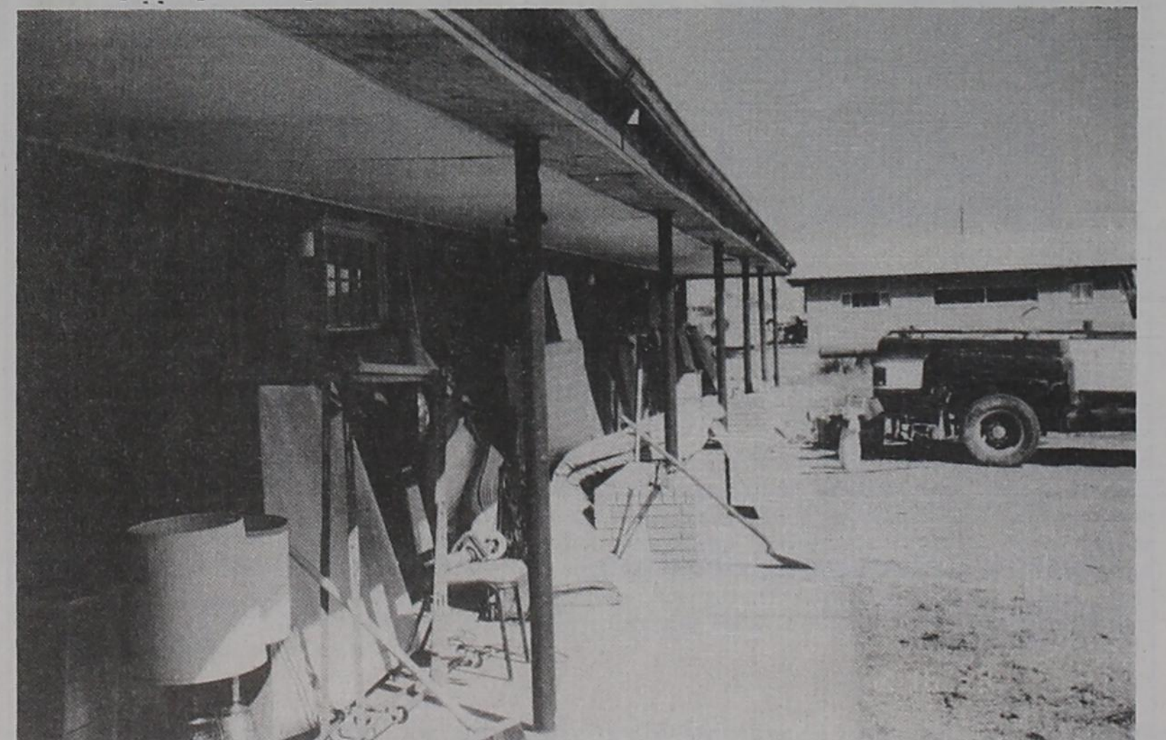
CLEANING UP THE SANDS....The Sands Motel on Highway 60 is finally getting a makeover, starting with a new roof earlier this year. Workers are now working inside and have moved room contents out to make room for painting and remodeling. ron carr photo
