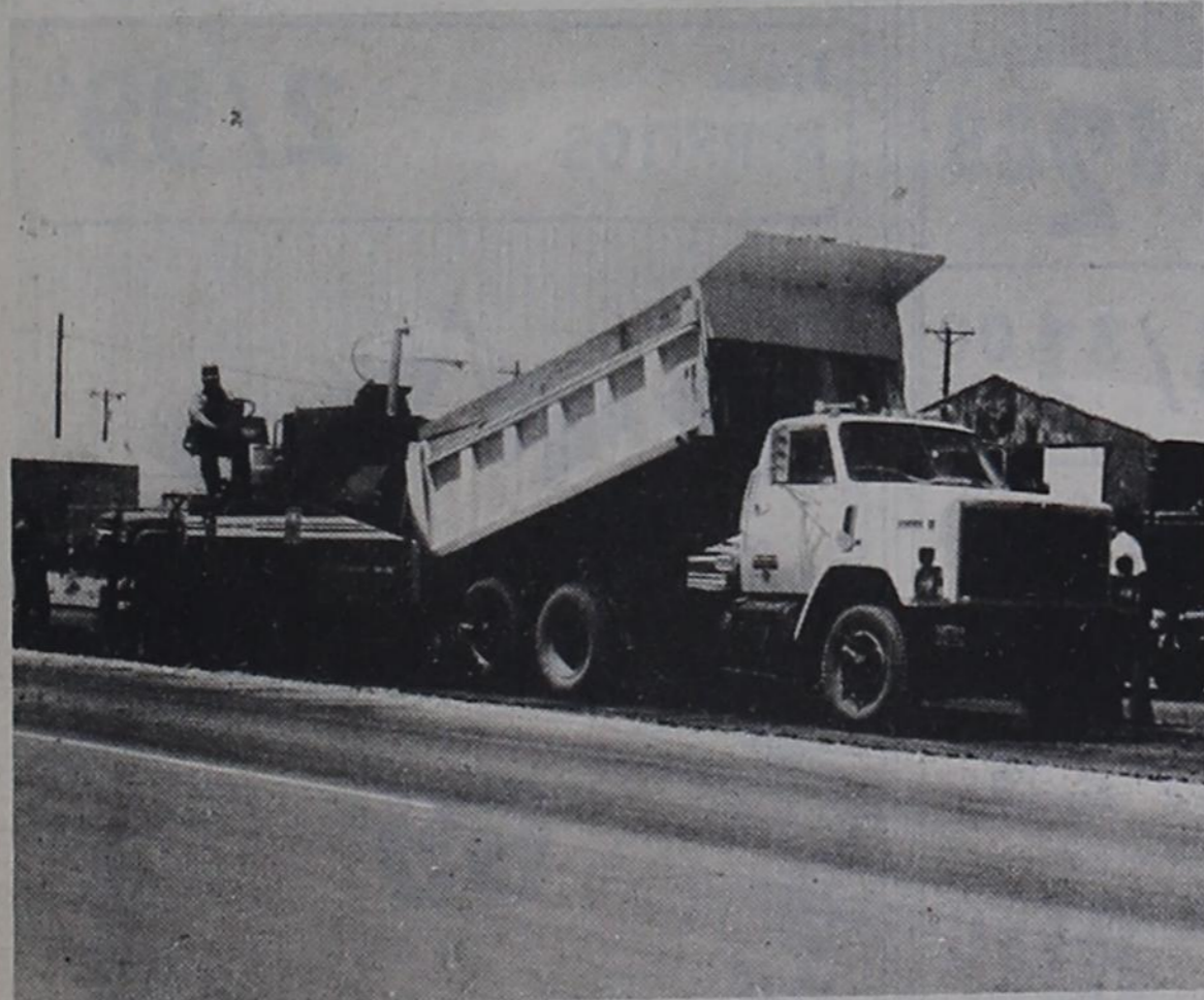
HIGHWAY WORK... The construction work on U.S. Highway 60 through Bovina continues to make headway.
