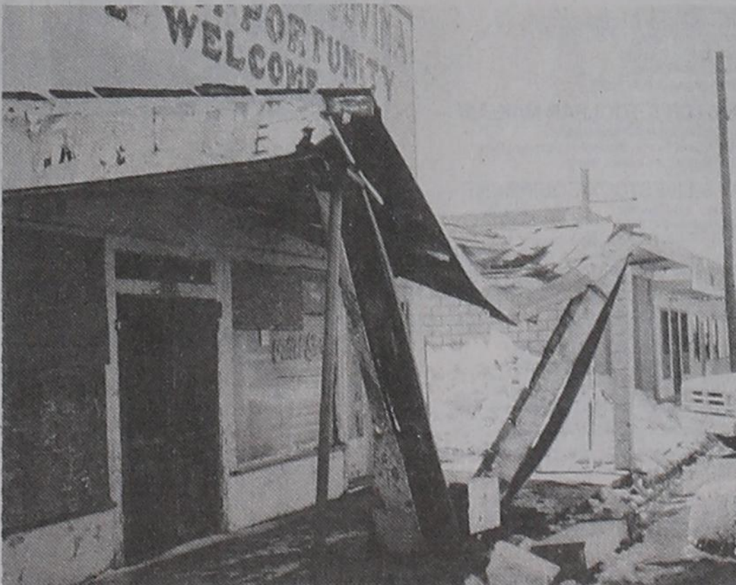
LANDMARK BITES THE DUST.... The heavy 13" snowfall last weekend in Bovina did not do a lot of damage around town. But on Main Street, the snow caused the awning of the old hardware store to collapse. ron carr photo
