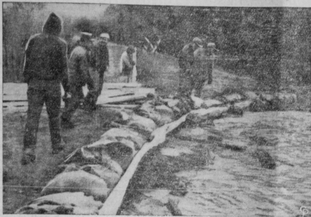
MISSISSIPPI RIVER ON A RAMPAGE —Farmers and National Guardsmen work desperately on a sagging levee in Meyer, Ill., but the flood-swollen Mississippi River was not to be held back. A few hours later, a ten-foot-high wall of water rolled over 80,000 acres of rich farmland. Thousands of residents had fled to higher ground before the river poured into their homes and barns. The breakthrough ended 24 hours of piling sandbags by the emergency workers on the crumbling levee.
