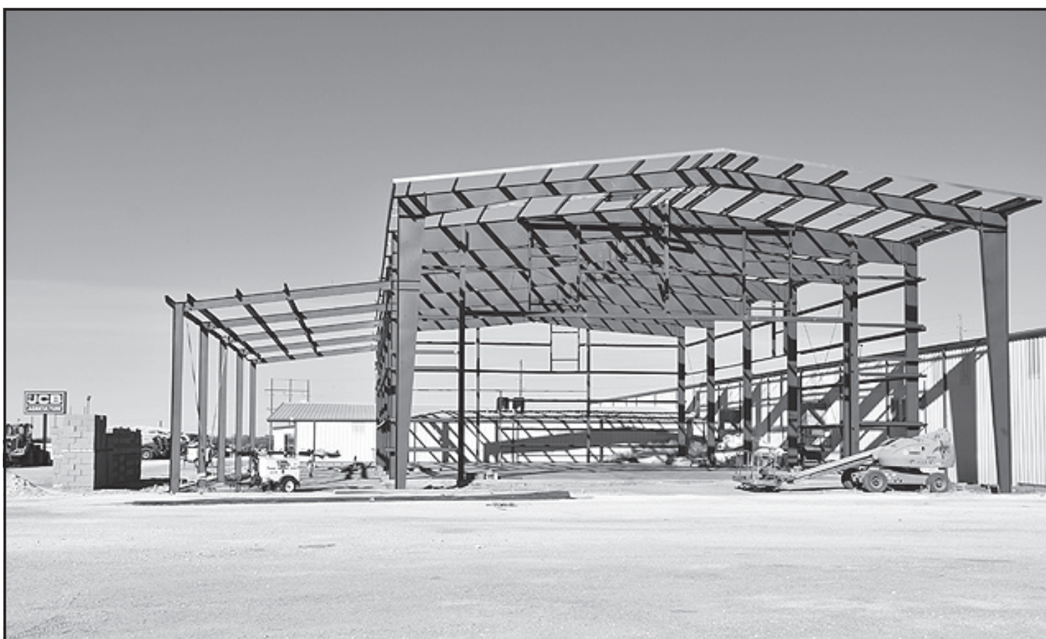
Construction is underway at Parmer County Implement Company. The expansion includes a new shop area and more storage space.
