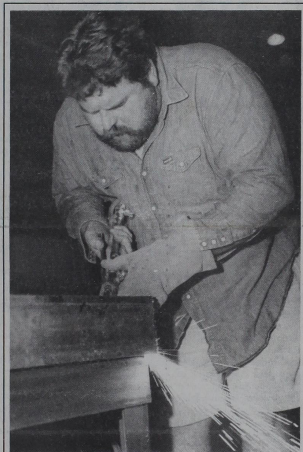
Sparkles JEREMY CHESNUTT: THE UNIVERSITY DAILY Fred Keotting works on one of the new handicapped areas for people in wheelchairs at the Lubbock Municipal Coliseum.
