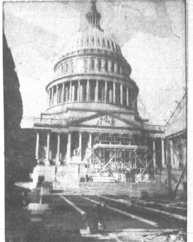
PREPARING FOR BIG DAY —Inaugural stand rises at Capitol, Washington, as preparations get under way for inauguration of Dwight D. Eisenhower as President, January 20.
