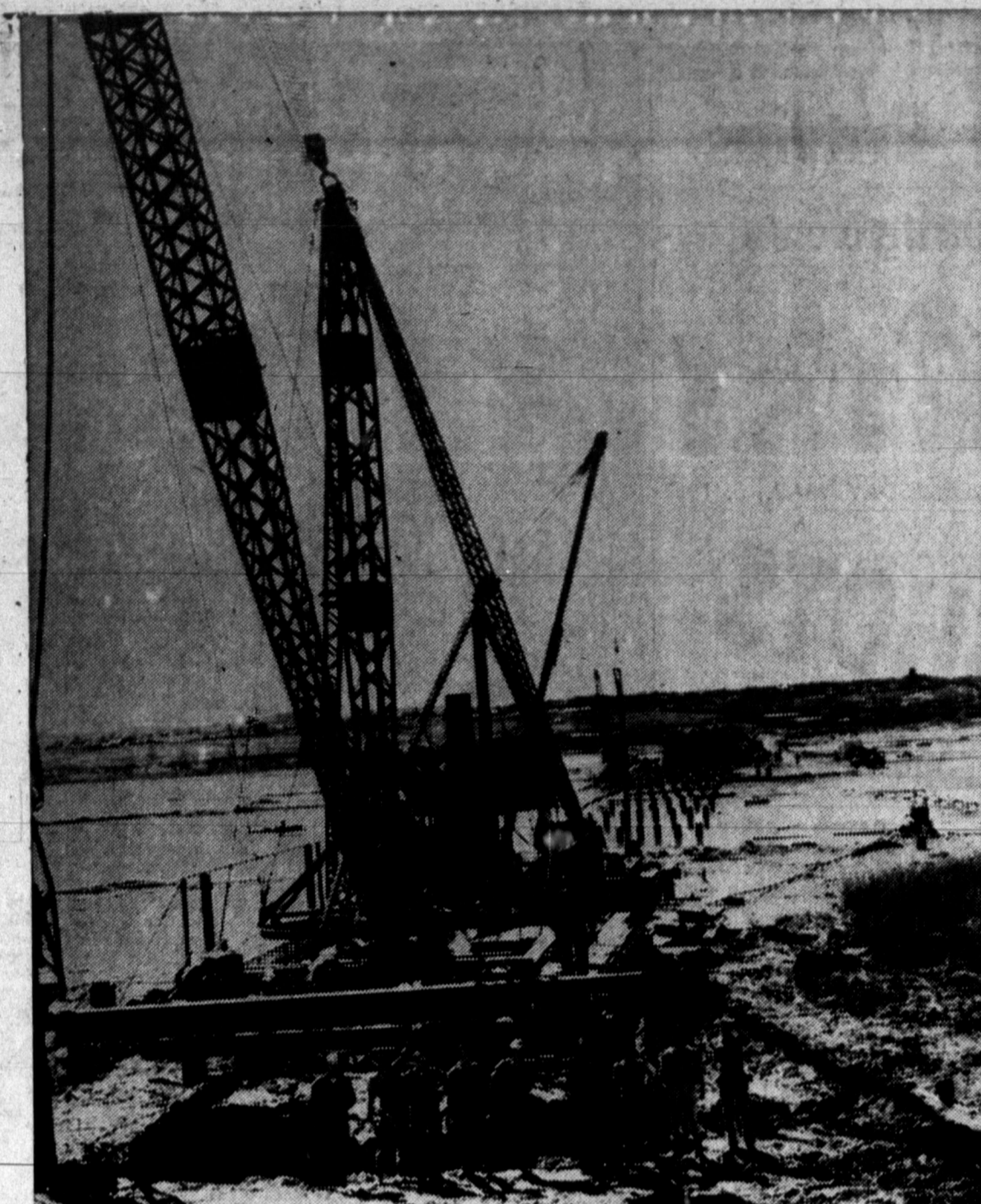
STAGE COMPLETED ON CANADIAN RIVER BRIDGE —Above is shown the pile driver crew just after the huge hammer fell for the last time on the last pile to be driven in the million-dollar highway bridge job on the Canadian river at Canadian. A portion of the old bridge may be seen at the right with the city of Canadian on the hill in the background. Crew members, left to right, are J. E. Menton, J. P. West, Ernest Adams, S. C. Tong, J. O. Roberson, R. T. Chalk, Joe Siddens, Wayne Baker and Supt. E. L. Boswell. On the platform are Marvin Horton and J. H. Hannon. All are employees of Austin Bridge Co. except Siddens and Baker who are inspectors for the State Highway Dept. See story on Page 1. (Rich Studio Photo)
