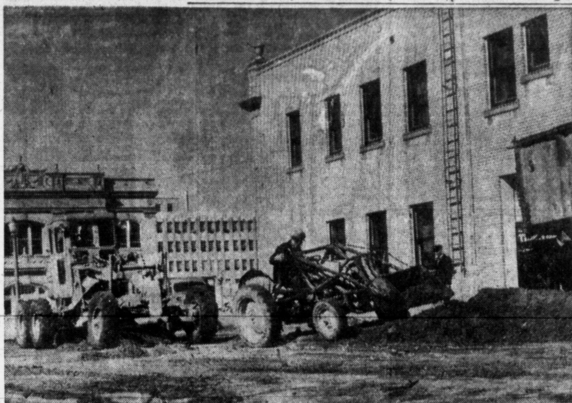
LEVELING OFF FOR NEW LOOK — Heavy machinery moved into the fire station property Tuesday to level off the property recently vacated by several trees which were removed by the city. The fire station is the second public building to be de-freed. County officials removed trees from around the court house last year. (News Photo)
