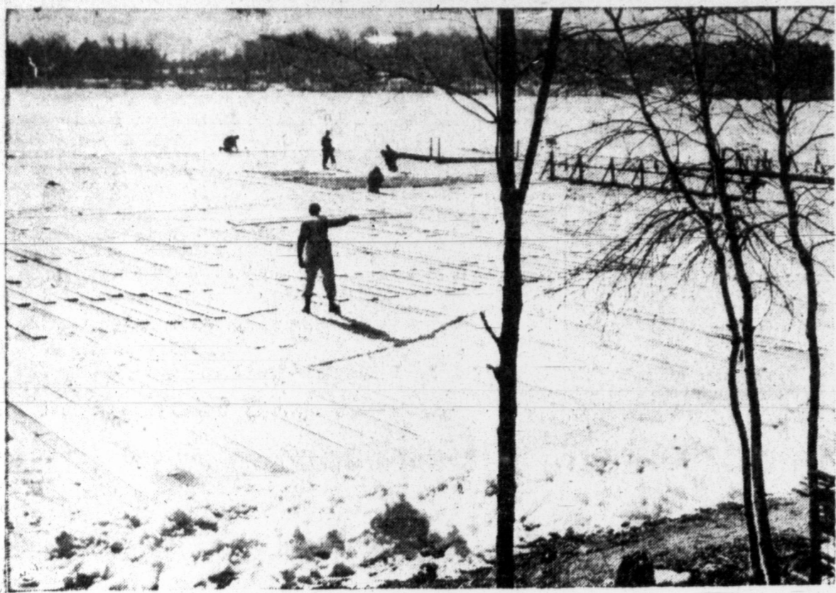
HOW TO FLOOR A SWIMMING POOL—These carpenters at Natick, Mass., are building a floor atop the ice on None Such Pond—and they're not as mad as you might think. The plan is this: They'll load the wooden floor with sand and when the ice thaws (they hope) boards and sand will sink neatly to the bottom of the pool, thus giving next summer's bathers a smooth, sandy bottom in place of the treacherous mud that has made swimming hazardous.
