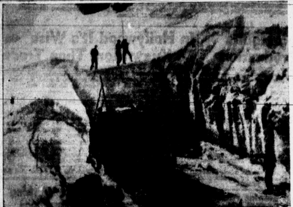
EXCAVATION IN CALIFORNIA—Road crews, working in deep crevice cut in the snow, prepare to dynamite more packed snow from U. S. Route 40 near Donner Summit, Cal. The scene is near where a crack streamliner recently was snowbound for several days.
