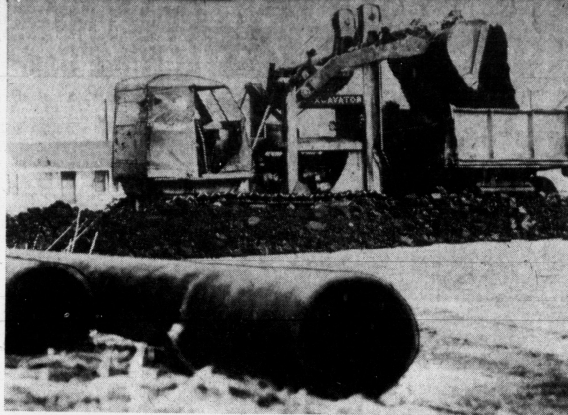
PRESSURE WILL BE UP —It won't be long until water pressure along Rham will be increased and with smooth riding paving to boot. Shown above is the city ditching machine going on the new bed for an eight-inch water main that will replace the old two-inch main running through that sector. The main will come off of a 10-inch main along Hobart. The new line will extend along three blocks of Rham, but only two blocks will be paved. (NewsPhoto)
