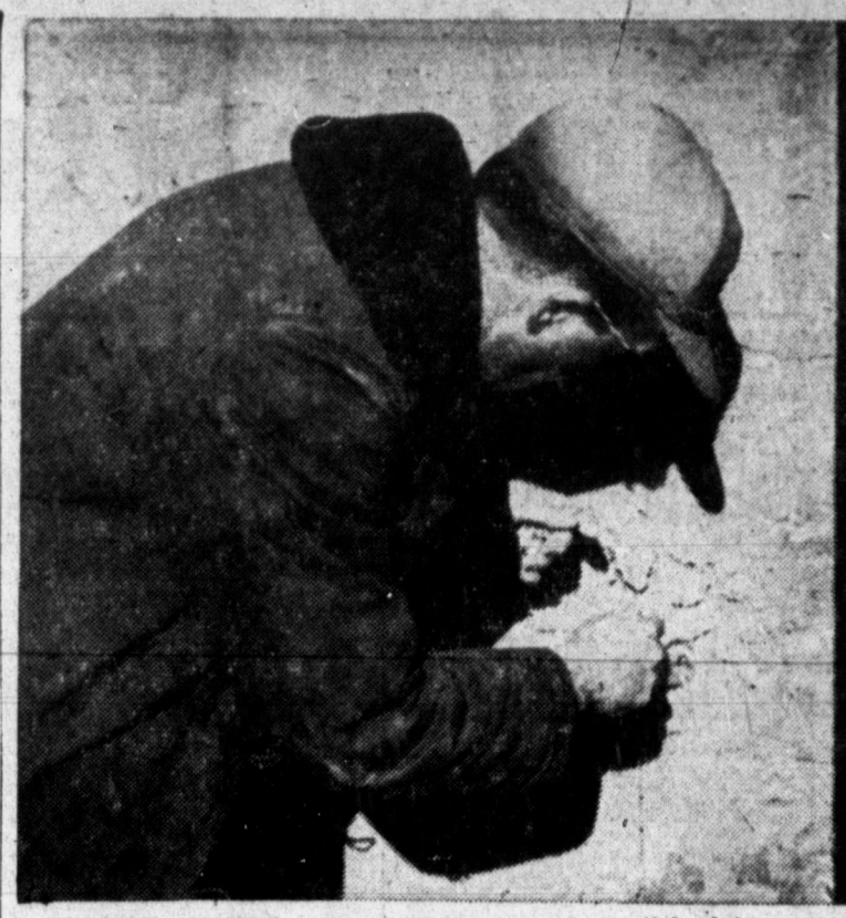
ELASTING CHUTE — Wayne Robinson packs a stick of dynamite behind the Pampa railway depot in preparation to blasting an old coal chute foundation in front of the railroad's roundhouse. Blasting began Thursday morning and continued through the afternoon. (News Photo)
