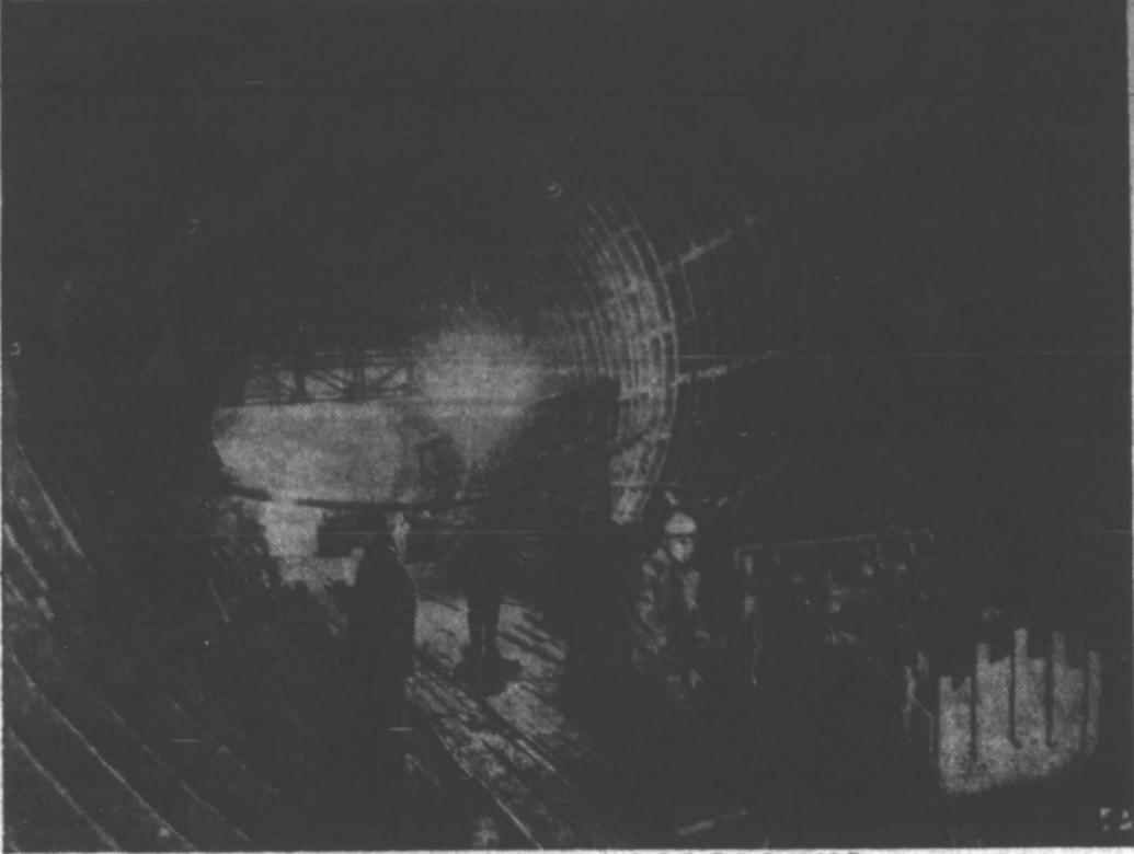
AT WORK IN THE RUSSIAN UNDERGROUND — Workmen labor under electric lights building the tunnel to the Byelorusskaya station in the Moscow subway system.
