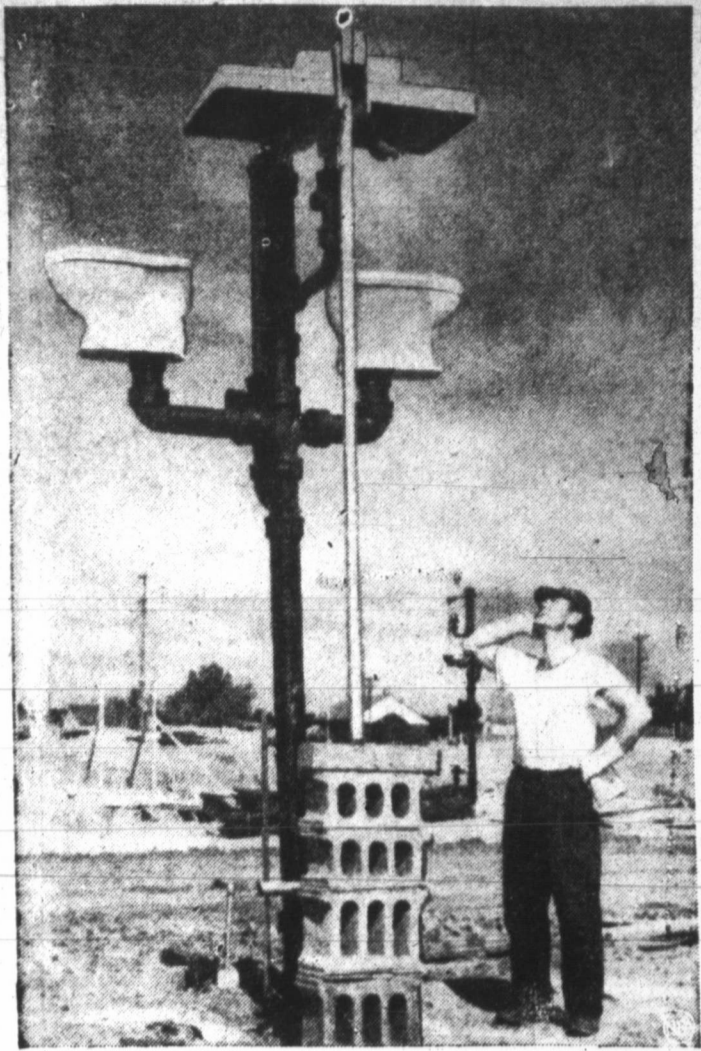
SEEMS PLUMB CRAZY —An unbelieving worker at site of a municipal housing development in St. Paul, Minn., stares at what appears to be outdoor indoor plumbing. Passersby at first thought it was something new in lampposts. Simple fact was that plumbers got ahead of carpenters and installed pipes and fixtures before the houses were up. There was some speculation on what would have happened if the roofers had gotten there first.
