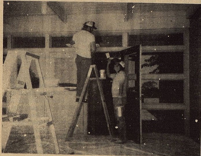
The R & M paint contractors are "hard at work" putting a new face on the school. Coach Roemisch & Coach Maxwell are really handy with a paint brush!
