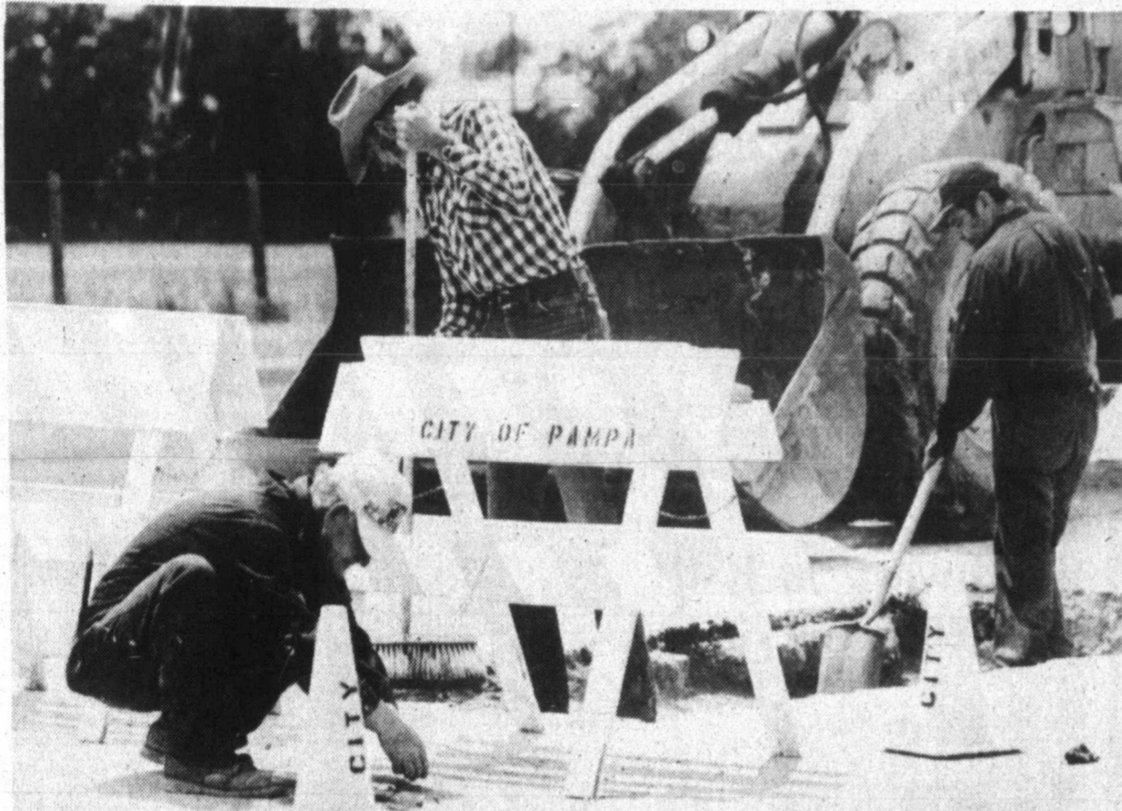
SPRING FIX UP work includes patching the street at Alcock and Hobart where a water line leak required removing the pavement to repair the leak. City workers from left, Leslie Edmondson, Alferd Oxley and Alferdo Compos are preparing to put new concrete on the intersection. (Staff Photo by Skyler Chapman)
