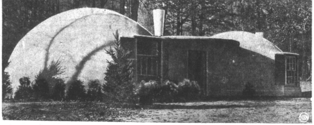
Igloo-like home is result of experiment in rapid building by spraying concrete mixture over large rubberized canvas balloons. RFC's Defense Homes Corporation is constructing the new type houses near Falls Church, Va.
