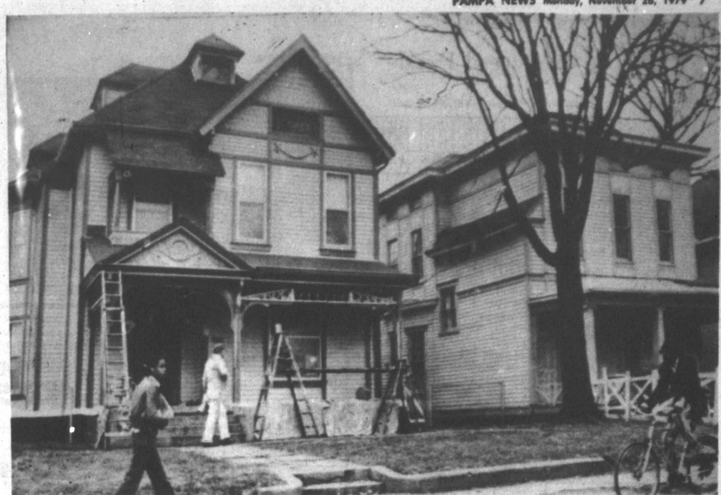
PAINTERS work to upgrade a historic house in 'old Northside' Indianapolis where preservation of the deteriorating neighborhood by the upper middle-class has displaced many of the elderly on fixed incomes and low-income families. (AP Laser photo)
