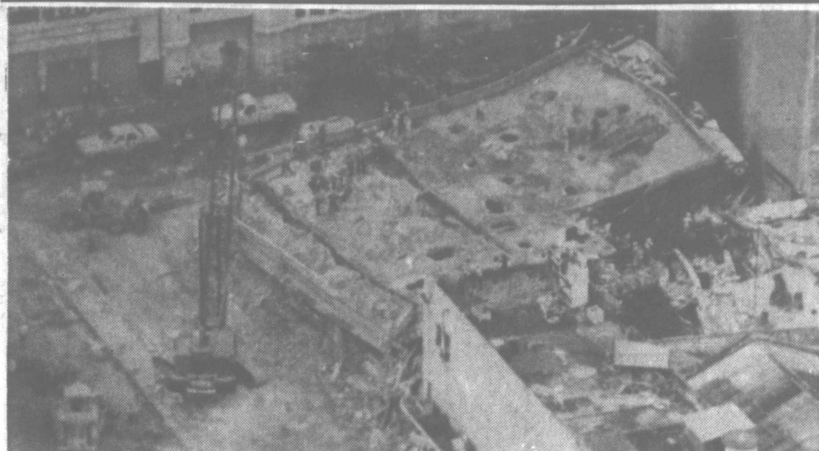
Rescue workers continue efforts Tuesday to find survivors in the Ruben Dario Building in downtown San Salvador.
