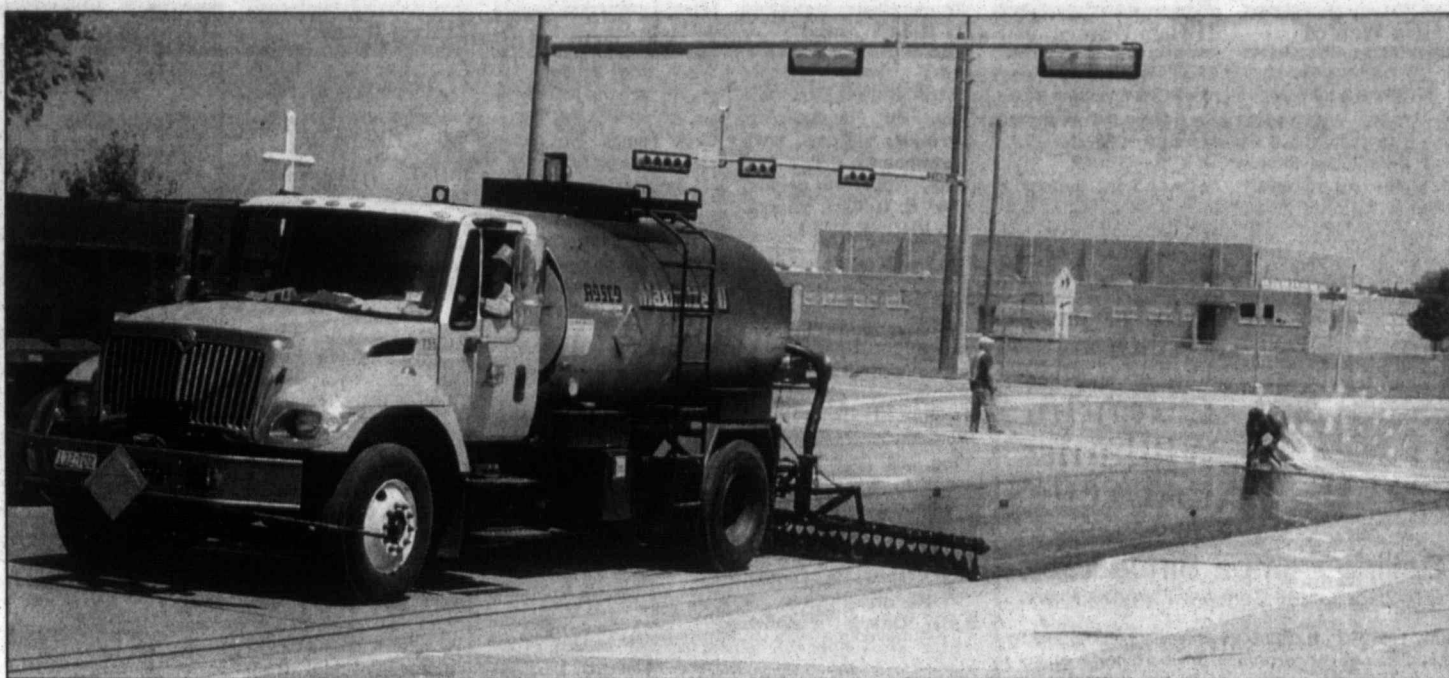
Hot tar is applied to 23rd Avenue between Hobart Street and Perryton Parkway earlier last week as work on seal coating 9.5 miles of city streets got under way after a brief delay due to rainy weather. The work is expected to be completed sometime this week.
