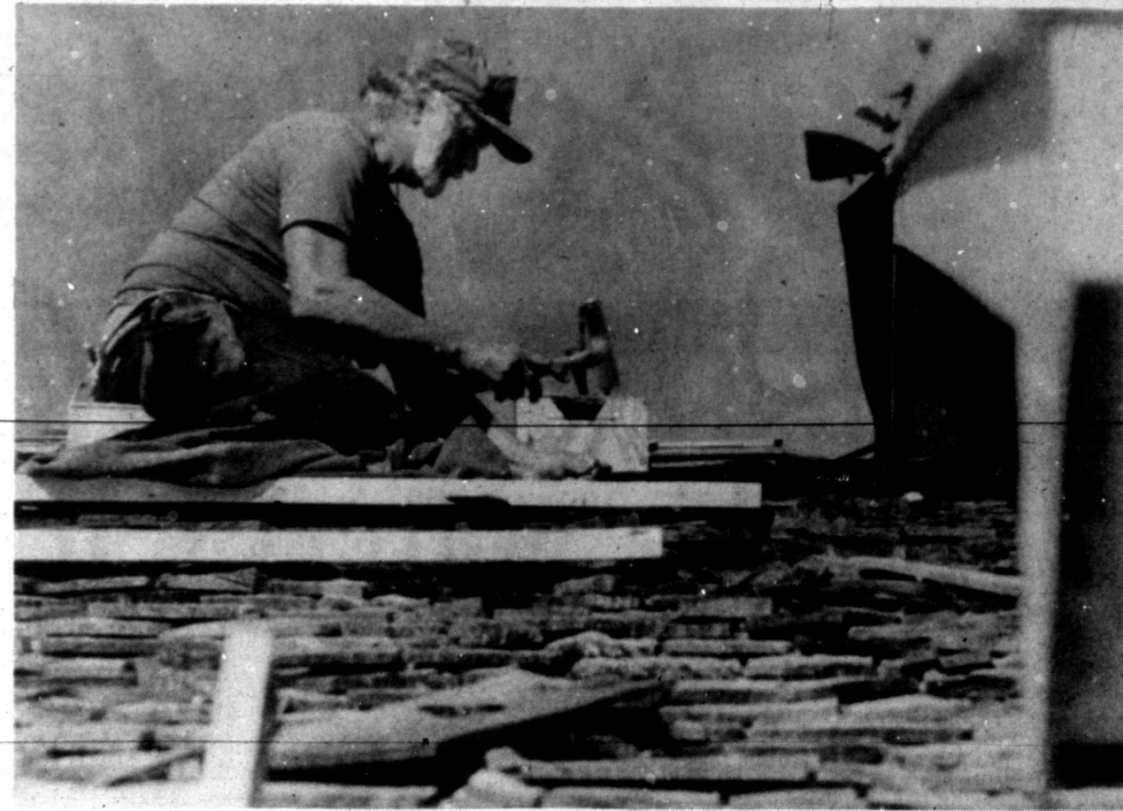
Mike Edwards of M & M Roofing applies wood shingles to a new house on Chateau Rue Drive in Pampa Wednesday. (Staff photo by Daniel Wiegers)
