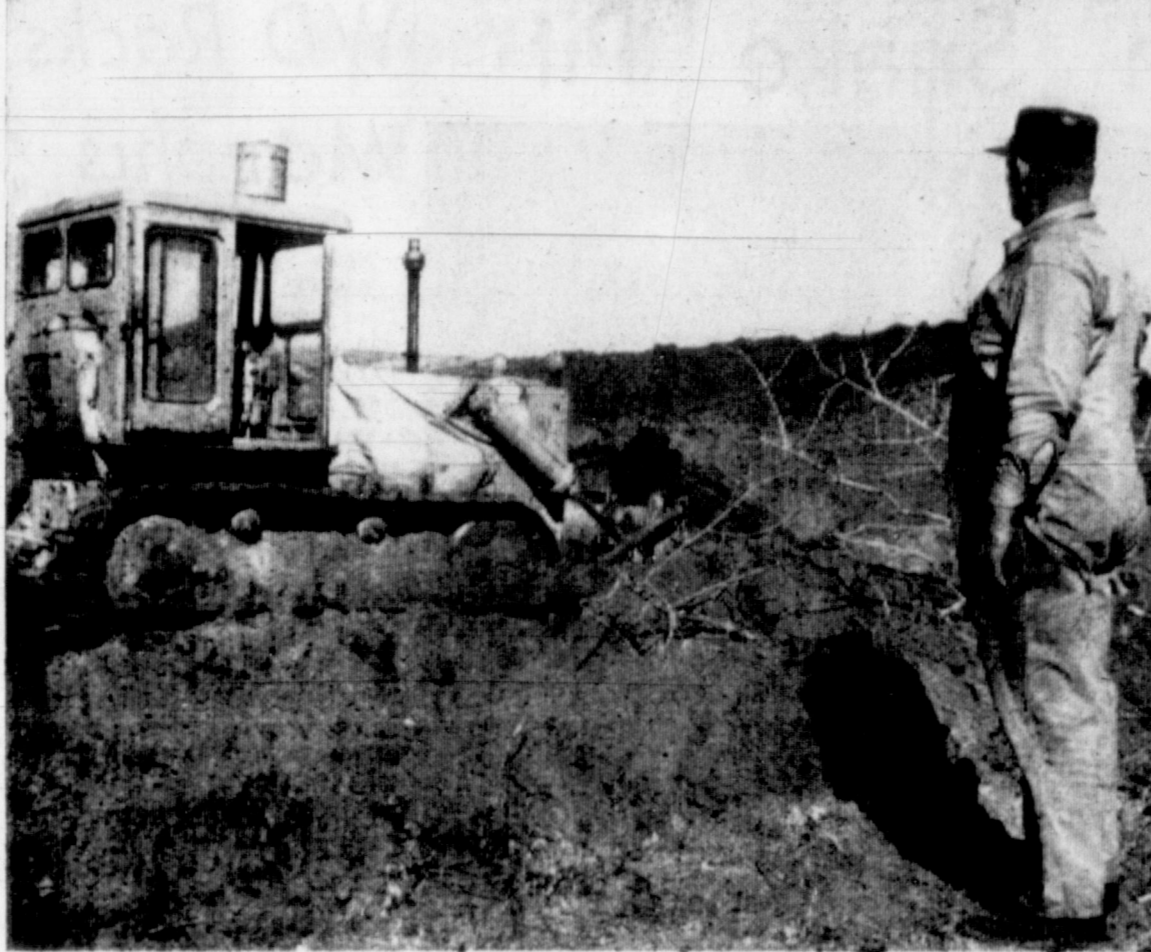
POND CONSTRUCTION — Grady Williams is shown observing construction of a pond on the R. W. Adams ranch, south of Kellerville. The pond is being constructed for better distribution of livestock grazing and to control water erosion. Williams plans to build three diversion terraces to control water erosion. (SCD Photo)
