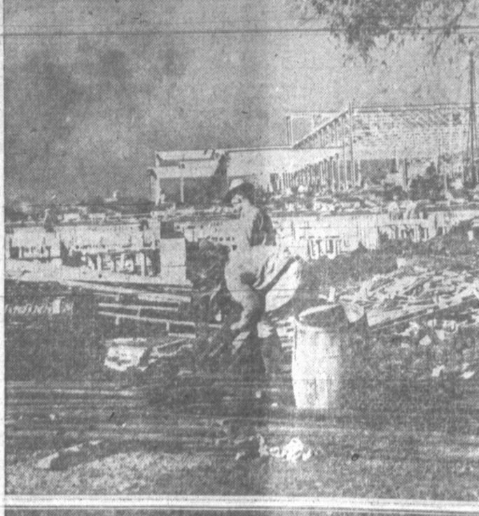
The steel frame of the $150,000 livestock building No. 1 for the Texas Centennial exposition at Dallas can be seen above as it rapidly takes form. With the $200,000 livestock building No. 2, soon to be started, it will house the state's exhibit of livestock in the nation's history when the exposition opens June 6.
