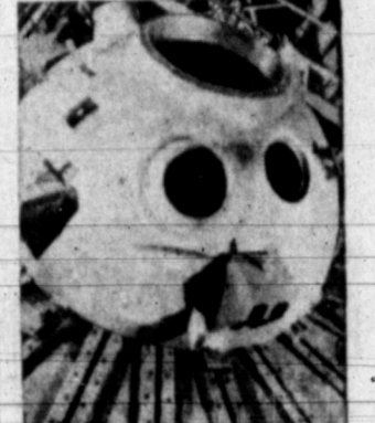
OLD NUCLEAR —Wide-eyed, pig-nosed chap with hole in head weighs 23 tons. It's the bottom section of a nuclear reactor vessel under construction in Milwaukee, Wis. Holets are for pipes and such.
