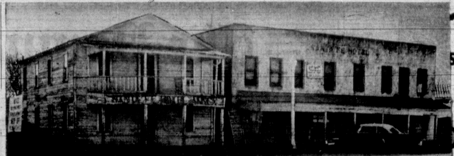
FROM OUT OF THE PAST — The Santa Fe Hotel and annex, looking much like the setting of a "wild west" movie, will soon be only a memory as workmen this week dismantle the 40-year-old building. When built in the early 1920's it was considered one of the finest build-
