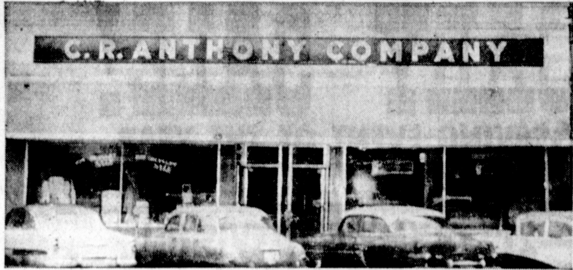
REMODELING COMPLETED — Shown above is the exterior of the C. R. Anthony store, 118 N. Cuyler, where remodeling work had just been completed. A new front, new lighting and other features to make the store better for the customers have been added. The local store was the 16th store built in the 244 store chain which covers 19 states. (News Photo)
