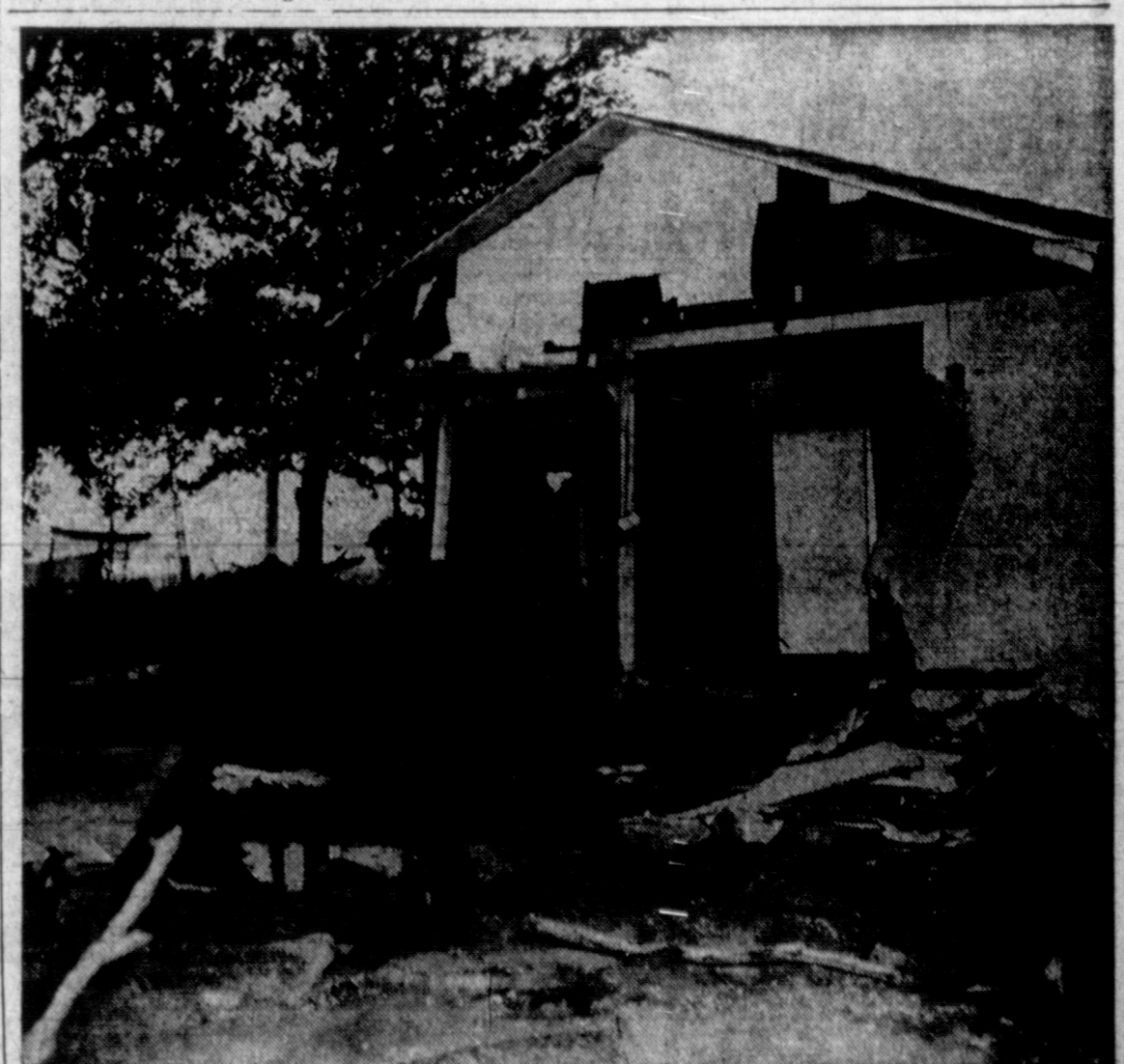
FLOODED HOUSE — Shown above is the Fred Browning home, 12 miles east of Lefors, after the Canton Creek, some 150 yards east of the house, flooded over the week end. The house was severely damaged and personal property damage was high. (News photo)
